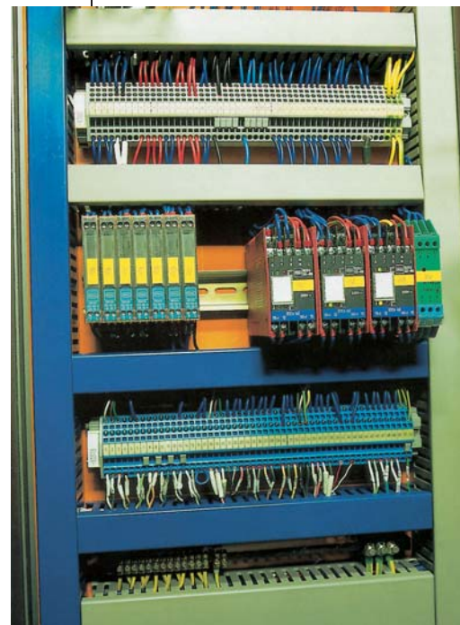
MCI-Switchboard with security barrier
